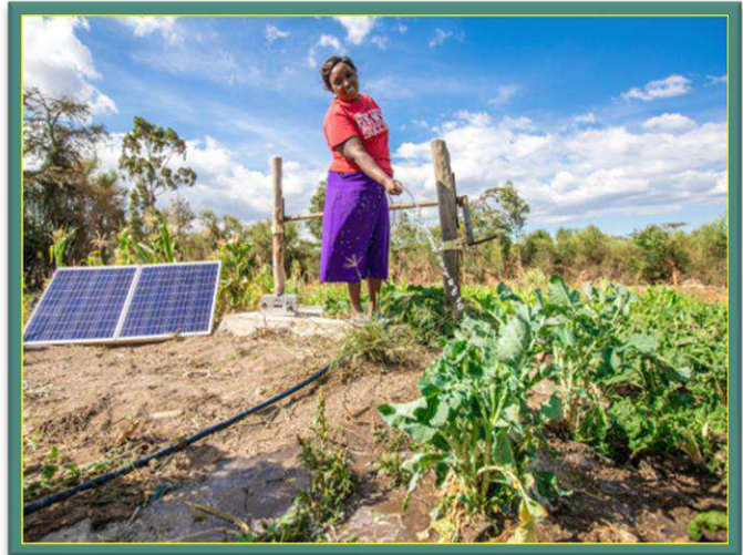
Photo 3: A small PV stand-alone system for less than 2 ha
