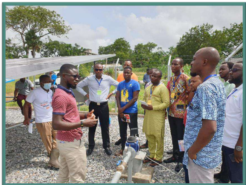
Photo 2 A solar-powered irrigation demo site at UENR, Sunyani
